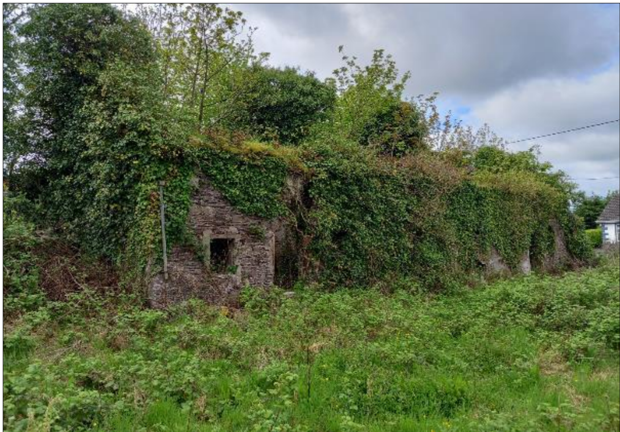
Plate 11.8: View of 19 th century vernacular structure extant in the western portion of the site
